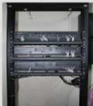
Newly installed PABX System
